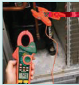
Dual Type K Inputs for taking differential temperature readings needed for superheat measurement
